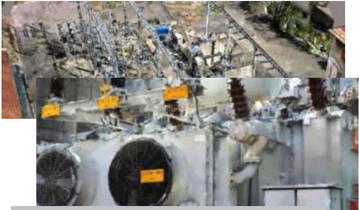
3D measurement of HV / MV sub-stations and thermography
